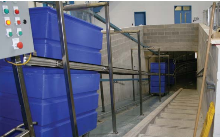
Laundry carts move on a conveyor through a cart washer and into a tunnel that transports them below the length of the plant from the soil side to the clean side. The system can transport 200 carts per hour.
