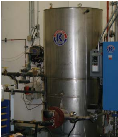
A water-heating system in the plant
