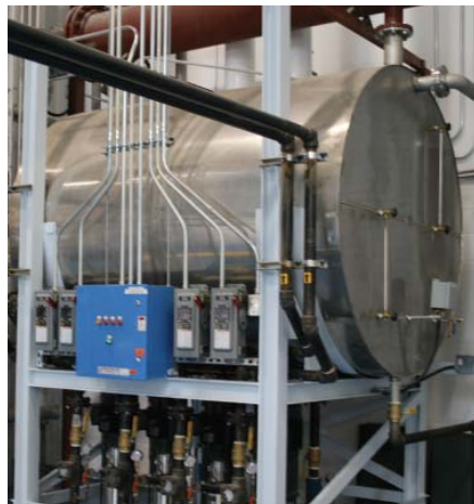
A hot water storage tank
