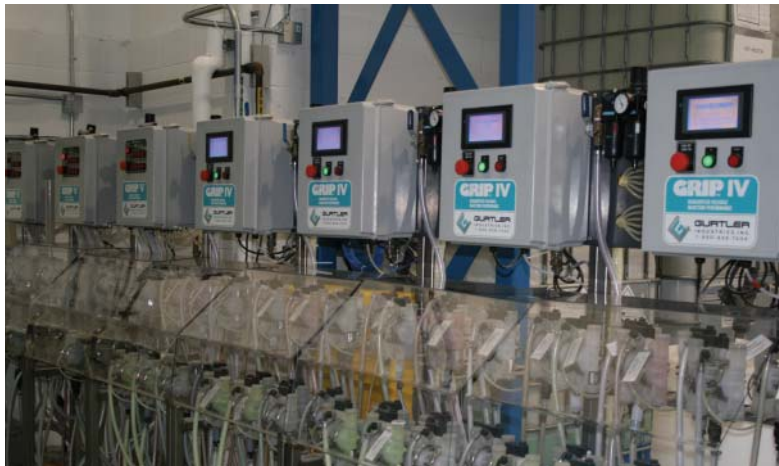
A view of the plant's chemical injection system
