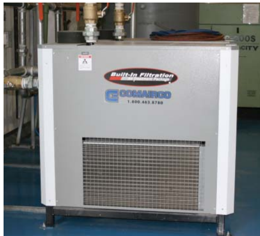
Air filtering machinery used in conjunction with the plant's air compressors
