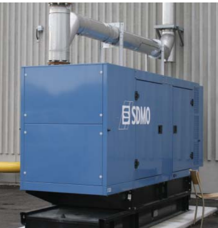
A backup electric generating system is available in case of power outages.
